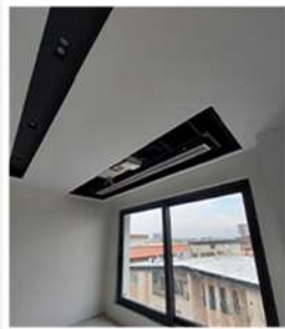
Access Panel Open
